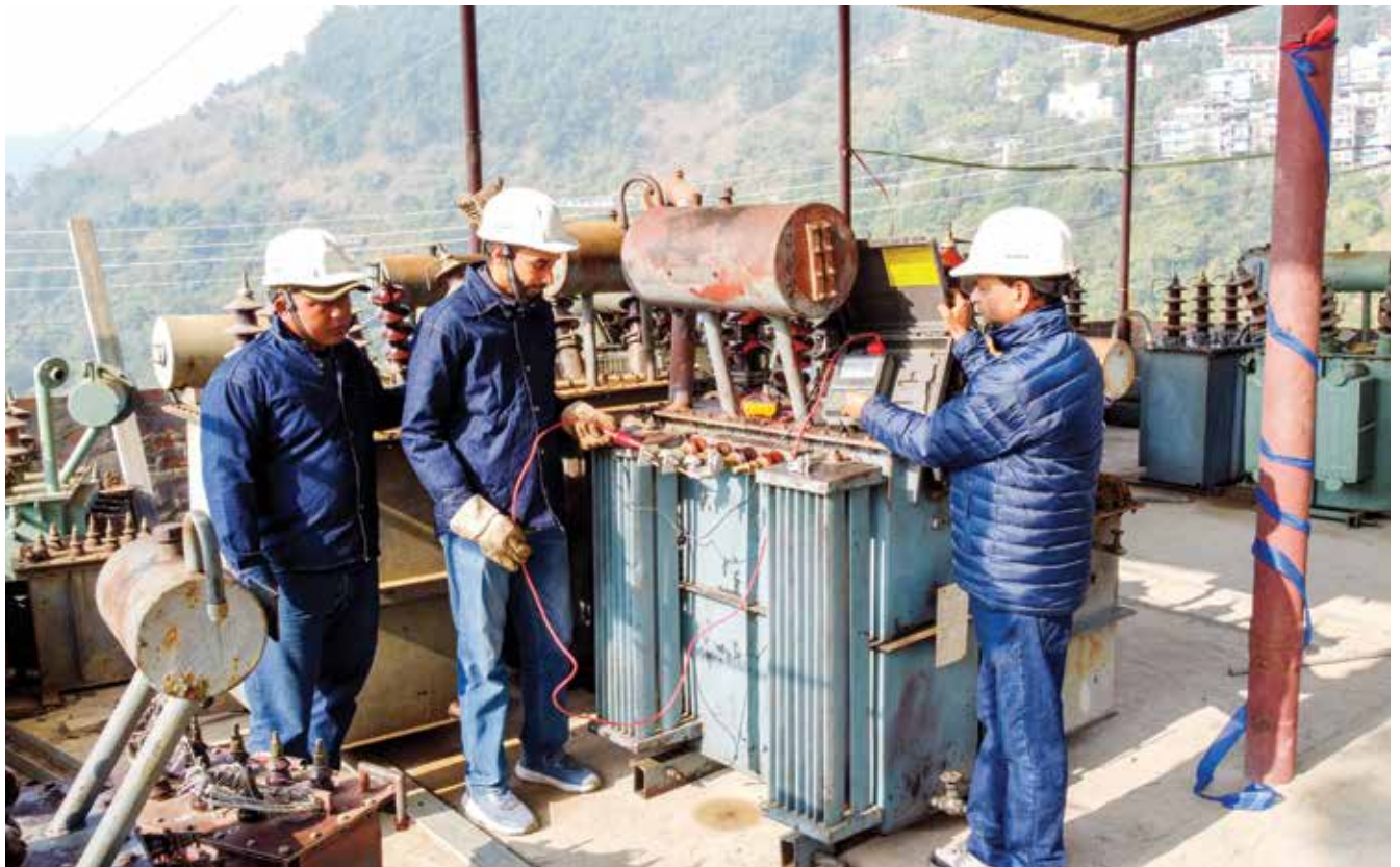
▲ Distribution Transformer Testing.
