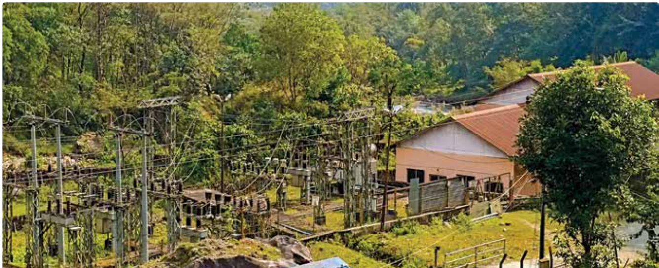
▲ 4 MW Khudi Powerhouse
